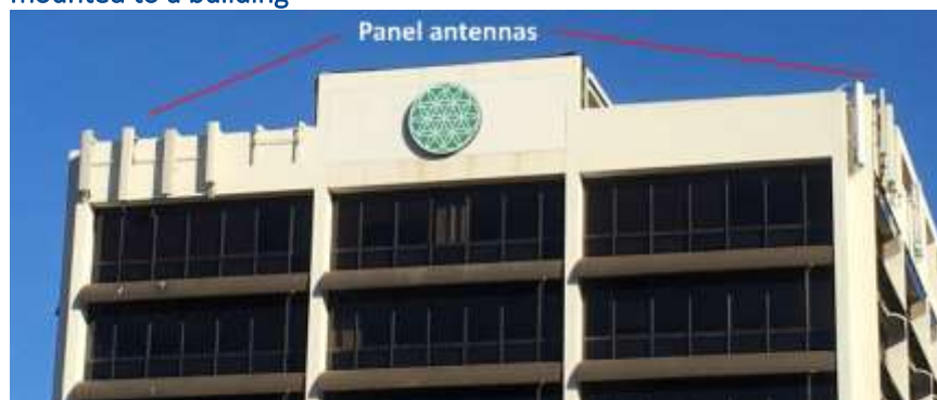
Figure 2: Low-impact mobile phone network panel antennas flush mounted to a building
