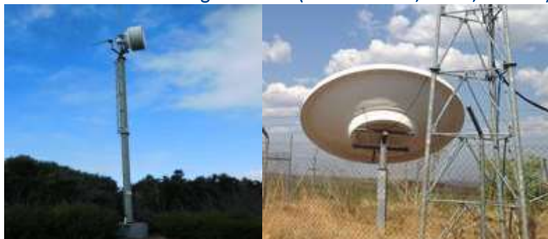
Figure 2: Satellite dishes for subscriber connection (LIFD Schedule, Part 1, Item 1A) (left) and radiocommunications dish for general use (LIFD Schedule, Part 1, Item 5A) (right)
