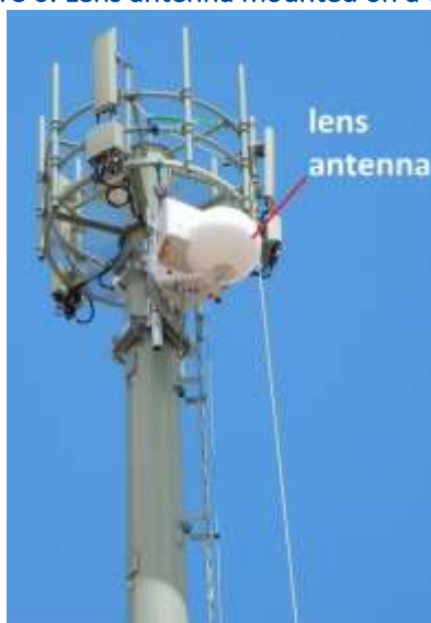
Figure 6: Lens antenna mounted on a tower
